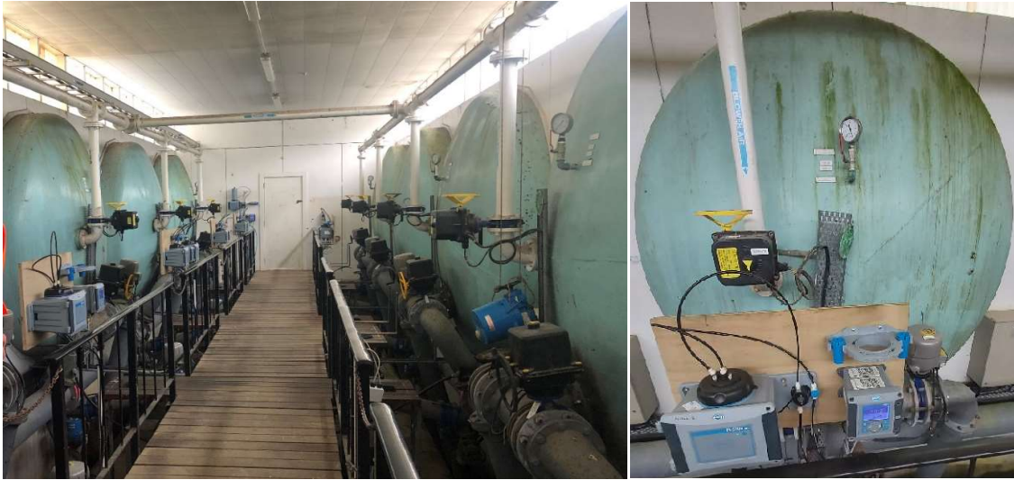
Figure 2: Pressure filters at Levin WTP
