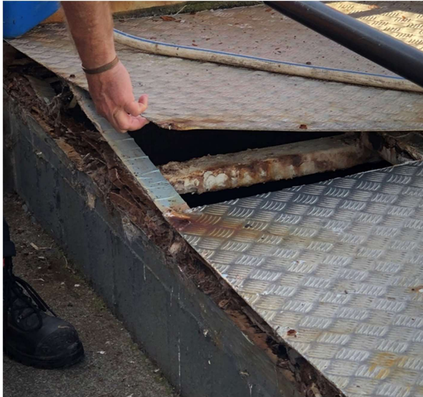
Figure 5: Deterioration of Sludge Storage Tank Roof
