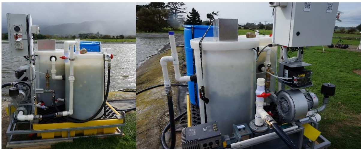
Figure 2: Pilot skid as installed onsite
